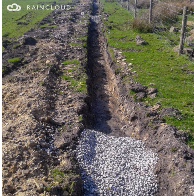
Plate 5: Check dam example
